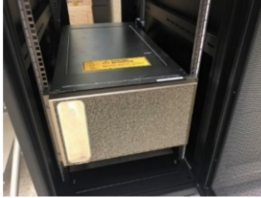
FIGURE 3. Installation of DGX A100
